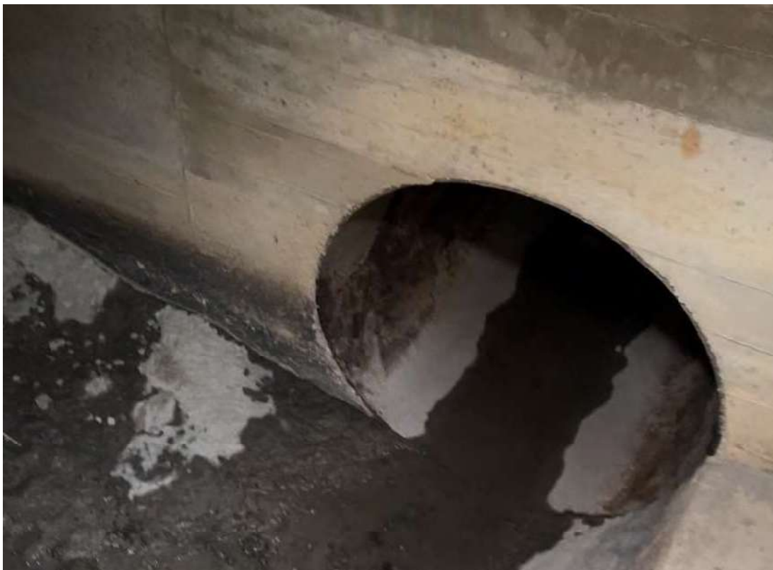
Photo A.4: Markham Road Culvert System 1050 mm Smooth Steel Pipe
