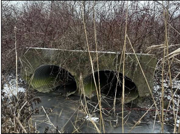
Figure 3-24: Outflanked and undermined twin CSP culvert with Concrete Headwall at downstream end of Reach MJC-2
