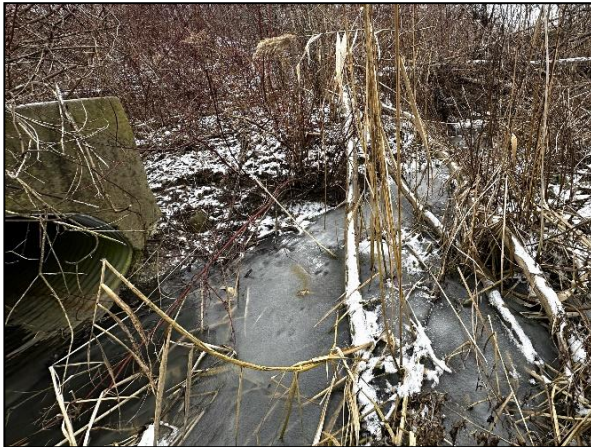
Figure 3-26: Tributary of Mount Joy Creek from the west at downstream extent of reach; contributing significant flow directed at the culvert
