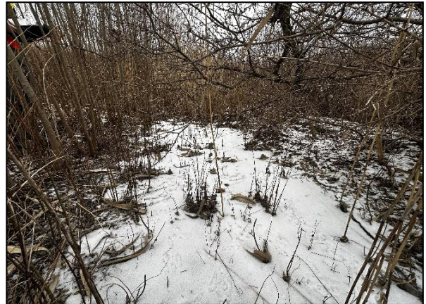
Figure 3-27: Mount Joy Creek upstream of the deteriorated twin culvert surrounded by wooded riparian corridor
