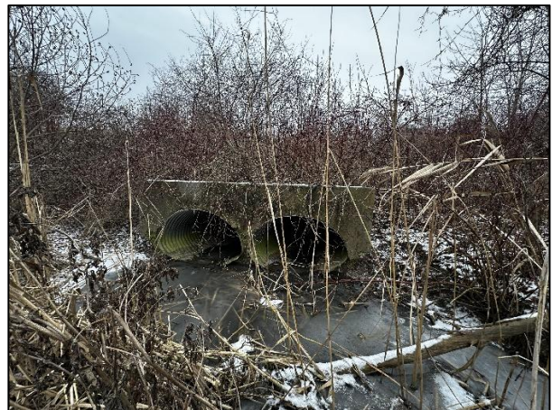
Figure 3-13: Deteriorated twin CSP culvert with concrete headwall at the downstream extent of the reach
