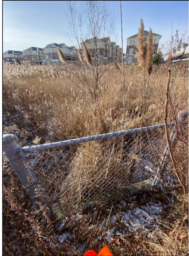
Figure 3-29: Looking downstream from the buried stormwater outfall at the aggraded and Phragmites infilled channel
