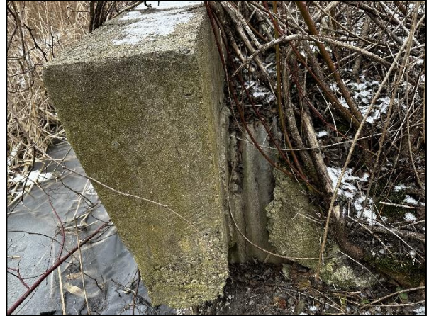
Figure 3-25: Exposed CSP and deteriorated concrete casing behind the headwall
